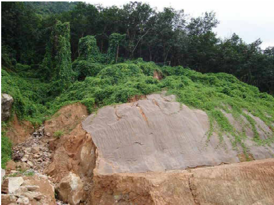
Picture 2 Failure of slope stability measures on the penstock route
