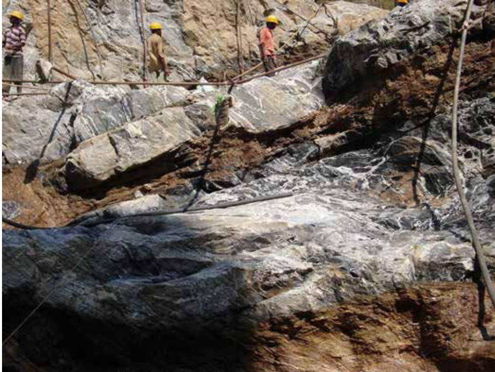
Picture 3 Power house excavations exposing the subsurface weathered seams within the hard rock in the Machine bay area.
